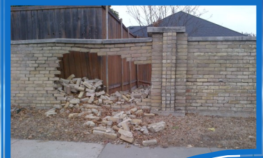
This photo was taken at Midway & Trinity Mills in December. We need to maintain and reserve funds for repairs in case of instances like this!
